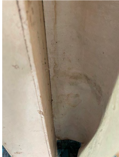
Photo 2. Staining beneath roosting bats in B2
